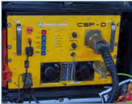
c) CSP-D2000 capacitor bank
